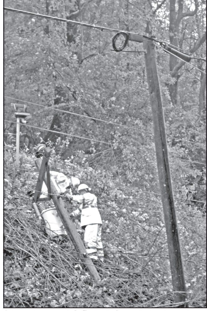
A downed power pole in Suches, being worked on by employees of the Blue Ridge Mountain EMC. Photo/Byron McCombs
